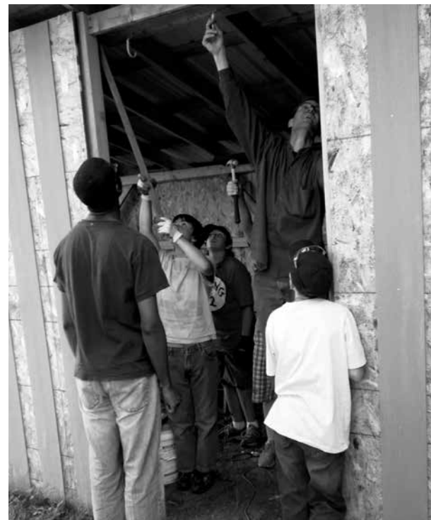
St Paul's Episcopal Church youth help Kelly build the new bike shed. Photo: Chelsea Froemke
