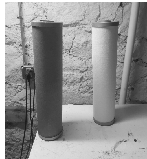
Whole-house lead water filter before and after replacement at Hannah House.
