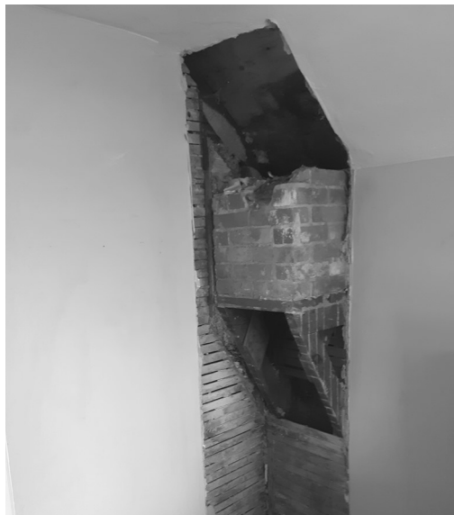
Surprise chimney remnants found in a wall while renovating a Hannah House bedroom.
