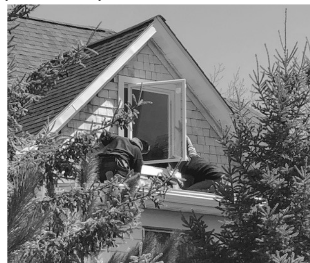
No more drafty windows on the 3rd floor of Dorothy Day House!
