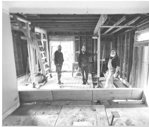
The beam. One of many structural improvements included in the Hannah House kitchen project.
